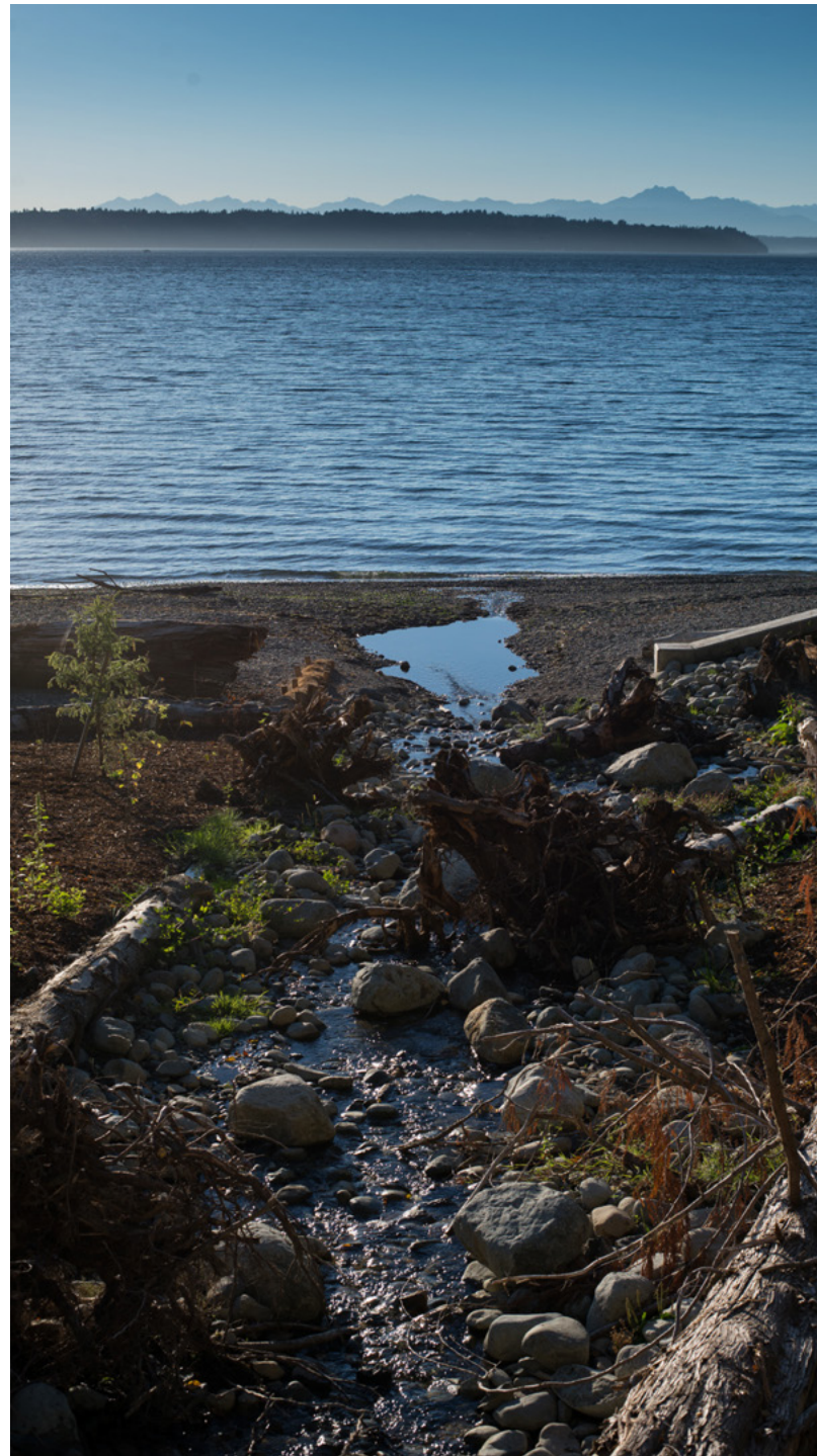
In Seahurst Park in Burien, Washington, a stream was restored by replacing a small culvert and fish capture structure that blocked streambed sediment from reaching the beach. The daylighted stream now delivers natural beach-material to sustain and nourish the restored beach on Puget Sound.
